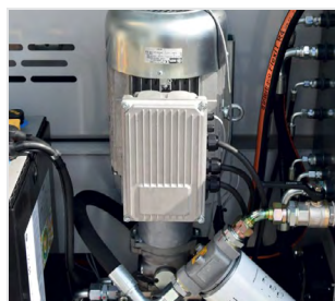
A/C electric power unit
