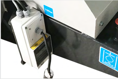
Thermal-magnetic switch panel and power line inlet.
